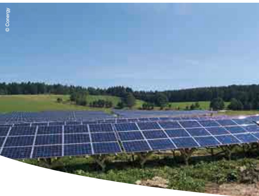
Large PV power plant
