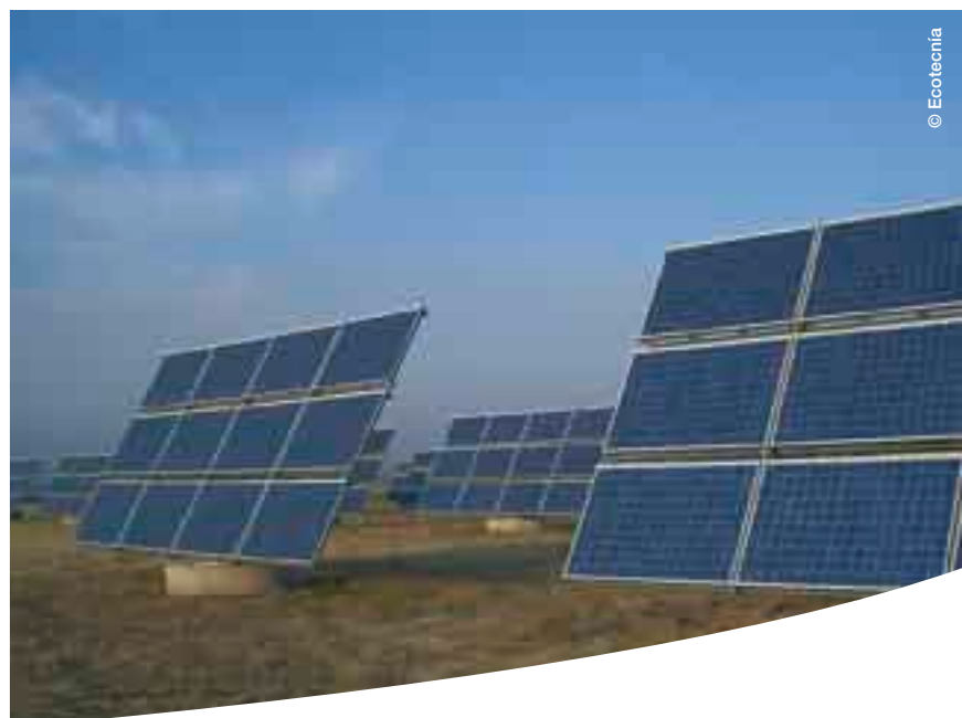
Large solar power plant in Spain
