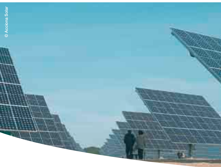
Large PV power plant with solar trackers located in Castejon, Spain
